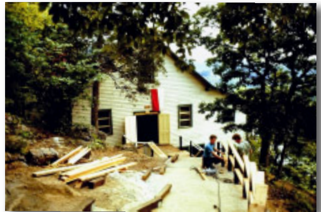
Last minute work on the latihan hall for Bapak's visit in 1970. (Photo by Rachman Cantrell)
